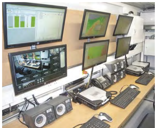
Operations centre in EWOC
