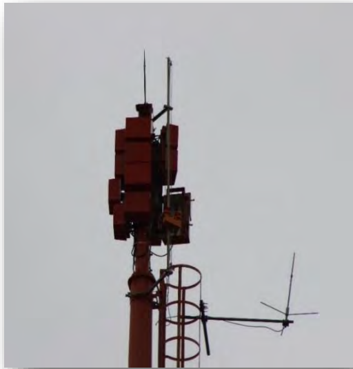
Example: Antenna – Empangeni, Durban - Horizontal Antennas
