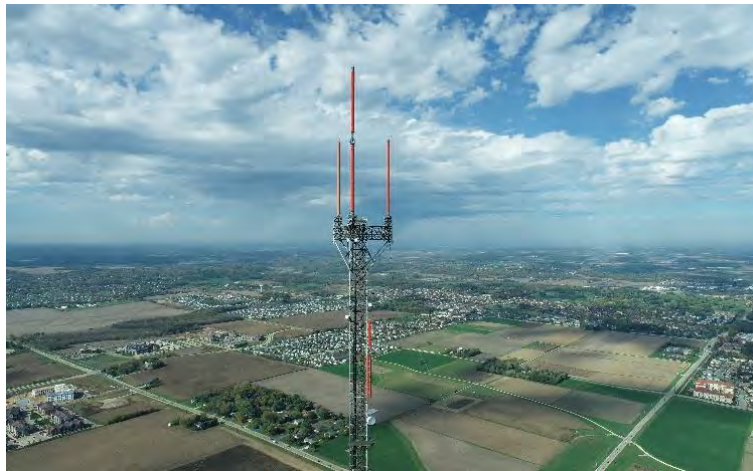
Above is a typical Antenna system installed at 470m AGL.
